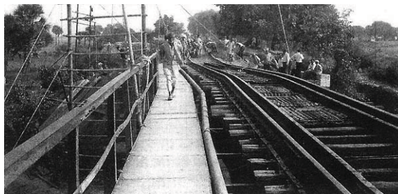
Fig. 18.19 Twisted rail line over a distressed railway bridge in Bihar caused by the subsidence of abutment and a pier (Pal, Roy, and Mishra 2009)
