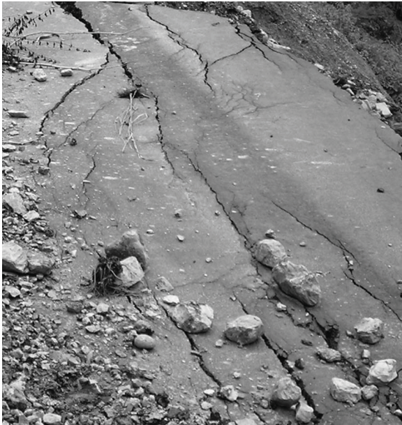
Fig. 19.4 Cracks developed due to passage of water into the subgrade
