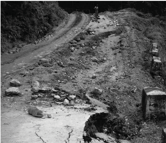
Fig. 9.10 Subsidence and deformation of road by seepage water beneath the road pavement and later vehicular movement in a highway in Darjeeling, West Bengal
