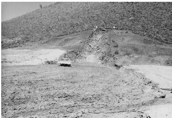
Fig. 14.29 An earth dam in Bihar showing partially compressed excavated hill slope material and earth
