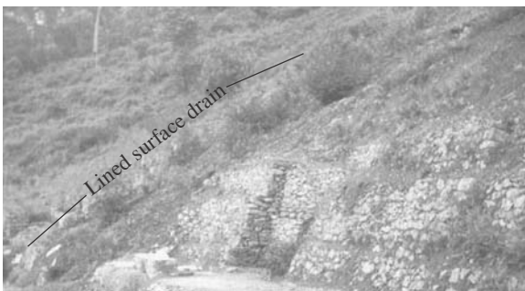
Fig. 21.24 Stabilization of slide-prone hill slope by drainage (lined surface drain) combined with re-profiling of slope by berms
