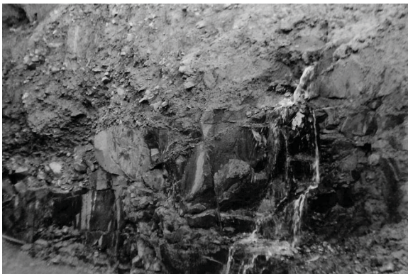
Fig. 9.7 Springs in weathered and fragmented rocks above a tunnel drift indicating seepage problem during tunnelling along the drift level
