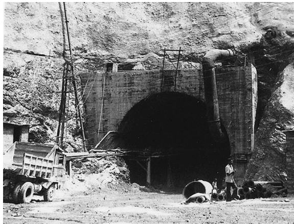
Fig. 16.18 A view of a tunnel at the construction stage showing pipe used for ventilation
