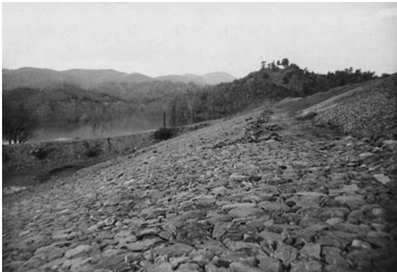
Fig. 14.25 Rip-rap constituted of slabs of hard and durable rocks covers upstream slope of an earth dam in Bihar
