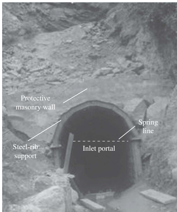
Fig. 16.2 Inlet portal of a horseshoe-shaped tunnel with steel rib support and a masonry wall to arrest debris slide
