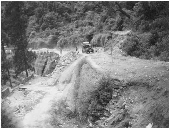
Fig. 21.18 Complex landslide (rock and debris slide) in Pagla Jhora in Darjeeling highway
