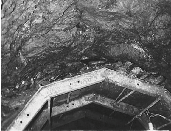
Fig. 16.5 Inside view of a tunnel showing deformed steel rib support due to overburden or rock pressure
