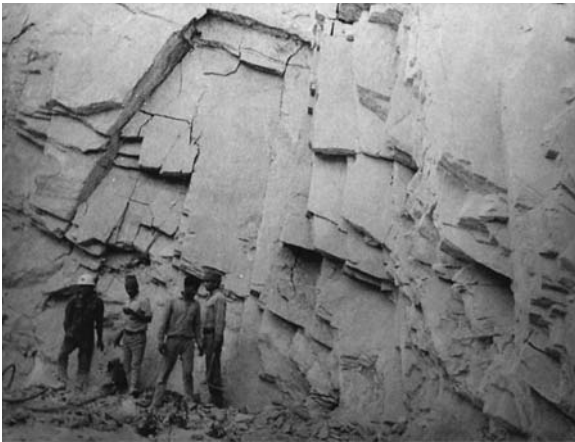
Fig. 3.33 Extensive joints (along strike and dip) in hill slope rocks along a highway causing rock fall and consequent road blockage
