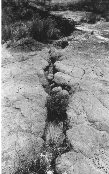
Figure 2.10b A tension crack running from an area that has subsided as a result of pillar failure, Witbank Coalfield, South Africa.
