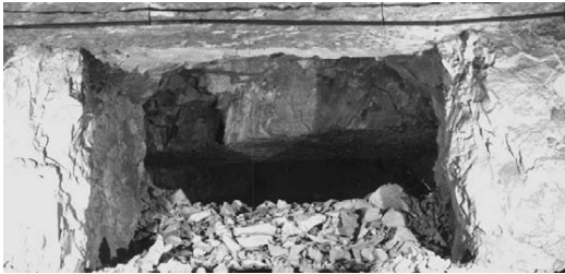
Figure 2.1d A pillar from the workings above punching through the roof of the workings below, in strong limestone of Carboniferous age, Middleton-by-Wirksworth, Derbyshire, England.
