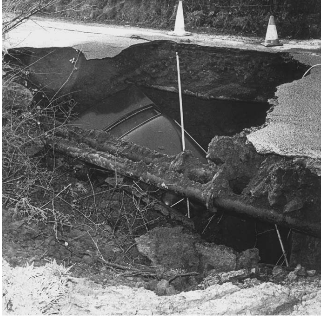
Figure 2.24 Collapse of an old shaft, trapping a car, Cardiff, South Wales.
