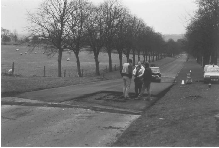
Figure 3.39b Road repair being undertaken to Wedgwood Drive following the reactivation of Crowcroft Fault in 1992. The fault scarps are visible in the grassed verge and fields to the left of the road.
