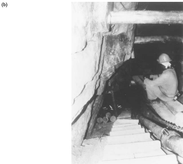
Figure 4.21 (a) Route of underground exploration of the Main Reef Leader. (b) Investigation of stopes via adit, Standard Bank site.
