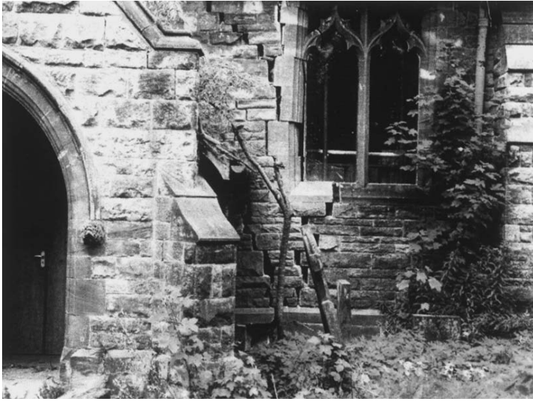
Figure 3.35 Damage to Barlaston Church caused by fault reactivation at a sandstone-mudstone contact.
