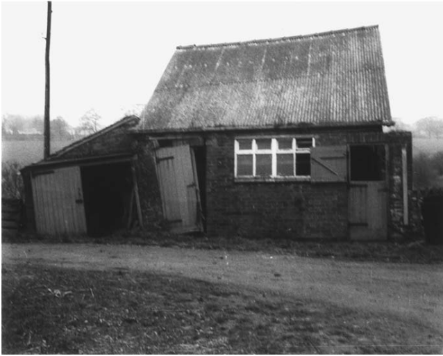
Figure 5.18b Severe damage caused to farm buildings due to subsidence caused by the abstraction of salt brine, Cheshire, England.
