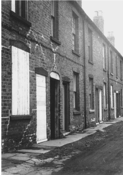
Figure 3.2 Examples of subsidence damage due to longwall mining of coal, Elsecarr, South Yorkshire, England, showing extensive cracking, walls being shored, and doors and windows blocked up after frames being severely twisted.
