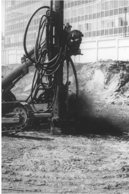
Figure 2.16 Probing for shallow old mine workings in coal with a rotary percussion rig, Sheffield, England.
