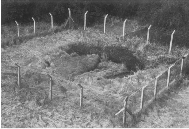
Figure 2.29 Collapsed mine shaft at Carrickfergus, Northern Ireland.
