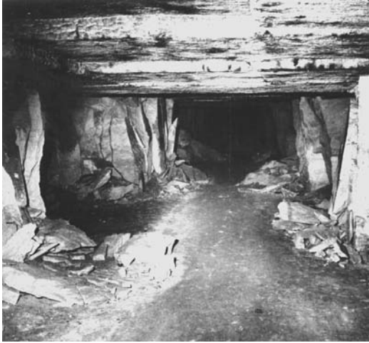
Figure 2.1c Spalling and partial collapse of pillars in the Bath Stone, old workings near Corsham, Wiltshire, England.
