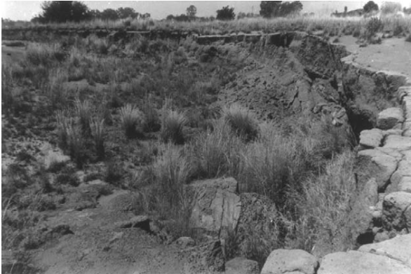
Figure 2.10a Subsidence at the surface caused by pillar failure in shallow abandoned workings, Witbank Coalfield, South Africa.
