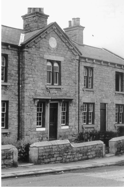
Figure 3.11 Subsidence damage in the neighbourhood of a fault step (windows fell out, door frames twisted and masonry severely cracked) Elsecarr, South Yorkshire, England. Fault step corresponds with dip in road.
