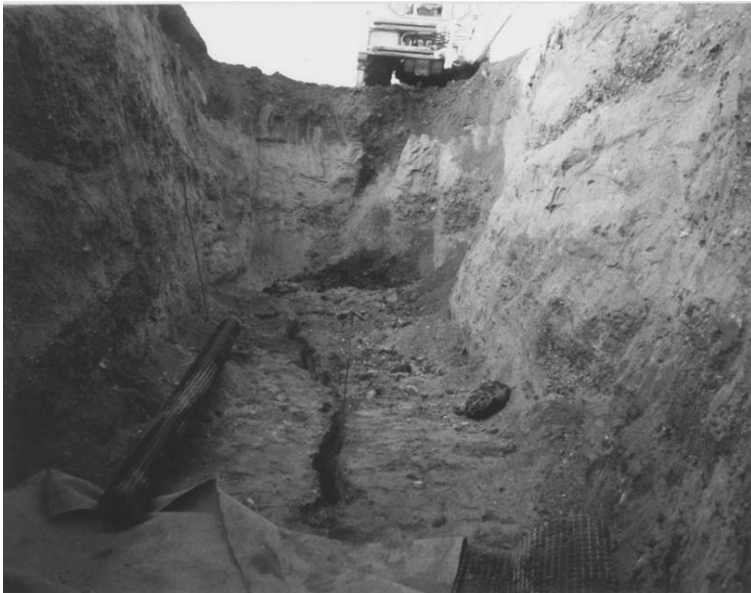
Figure 3.40 Reactivated fault exposed in a trench on Downes Bank. The trace of the fault is marked by a ground fissure about 0.1 m wide. Remediation of the fault was to be made using a geotextile mat and granular fill.
