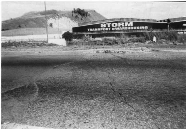
Figure 4.12 Subsidence on a faulted dyke contact leading to cracking of ground.
