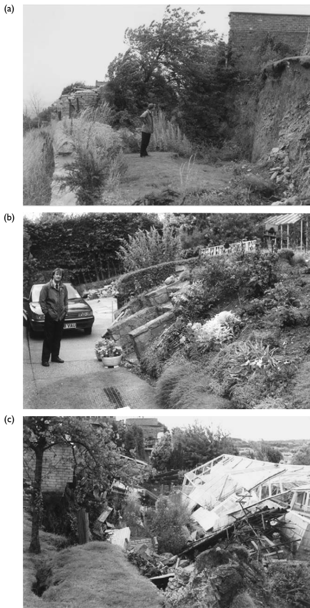
Figure 10.17 (a) The backscarp of the mining-induced landslide at Bolsover, Derbyshire, England. (b) The upheaved toe of the landslide at Bolsover, now landscaped. (c) Structural damage to a perimeter garden wall and a greenhouse at the crest of the Bolsover landslide.
