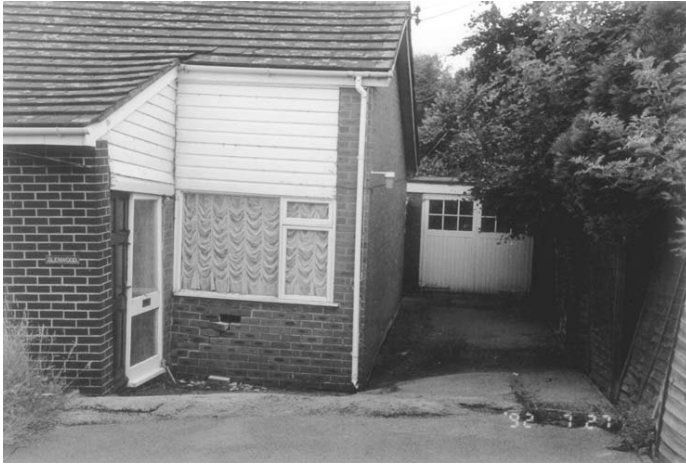
Figure 3.38b Reactivation of the Crowscroft Fault, Longton Road, Barlaston, causing damage to a house, the fault scarp running immediately in front of the house.
