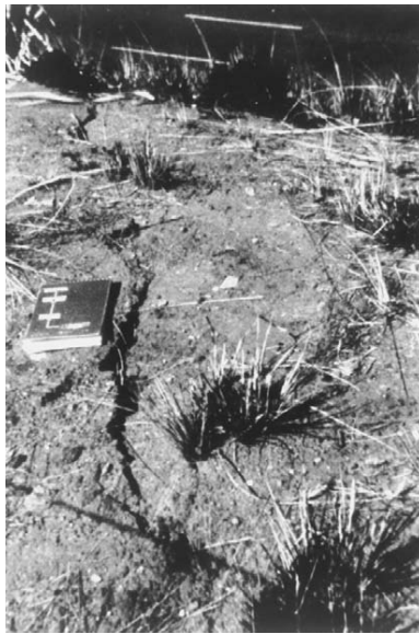
Figure 4.25 Cracks developed on the north bank of the M2 motorway due to subsidence.
