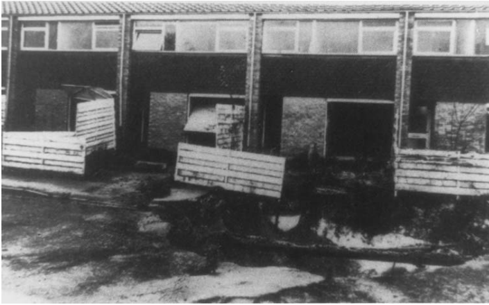
Figure 2.7 Collapse of shallow workings in chalk at Jacqueline Close, Bury St Edmunds, Suffolk, England, the Close ultimately was abandoned.
