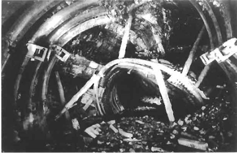
Figure 5.1 Large displacements around an originally arch-shaped coal mine access tunnel (from Pan, 1989).
