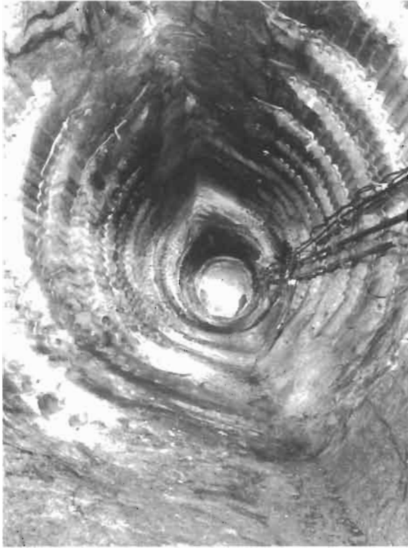
Figure 2.7 Tunnel deformation caused by high rock stresses at the Underground Research Laboratory, Manitoba, Canada.
