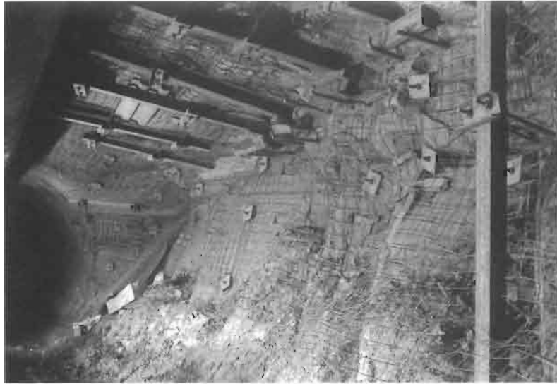
Figure 2.6 Tunnel in mudstone which has deteriorated over a period of several years after excavation.
