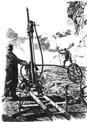
(b) Mounting single rock drill on Track. First step towards mechanization. Note improved working conditions.
