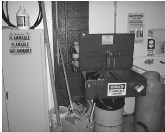
FIGURE 7.50 Obstructed access to extinguisher.
