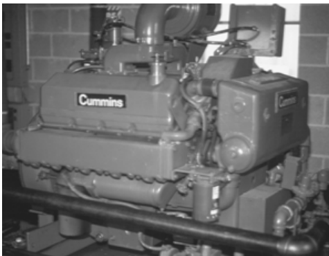
FIGURE 6.70 Fire pump, diesel.
