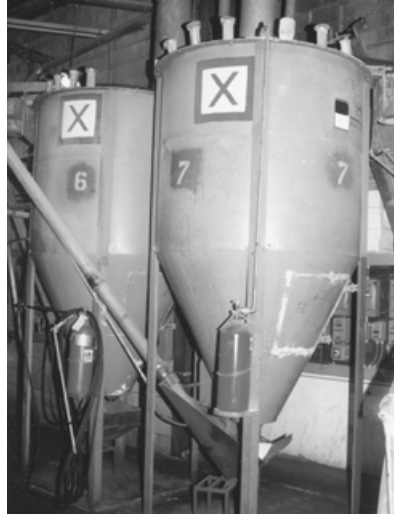
FIGURE 6.88 Manual carbon dioxide system.
