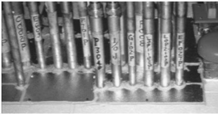
FIGURE 6.4 Fire barrier around conduit.
