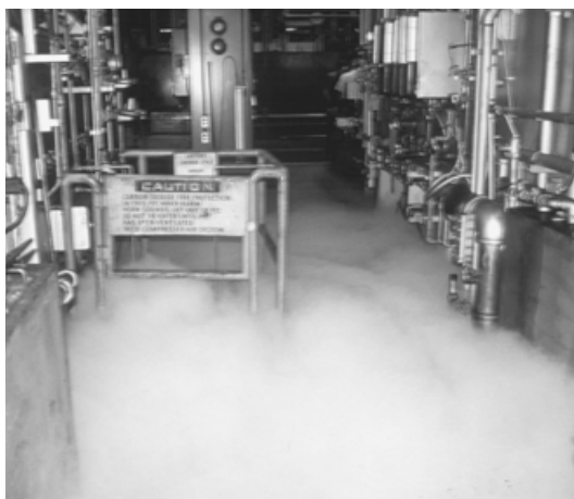
FIGURE 6.92 Carbon dioxide accumulated at floor level.
