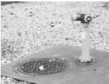
FIGURE 6.74 Fire department connection.
