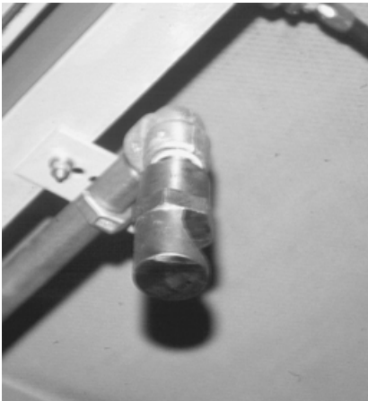
FIGURE 6.94 Halon system nozzle.
