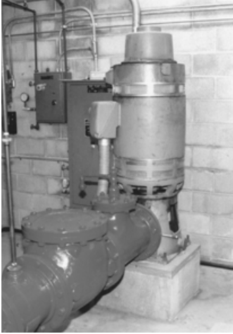
FIGURE 6.72 Fire pump, electric, vertical shaft.
