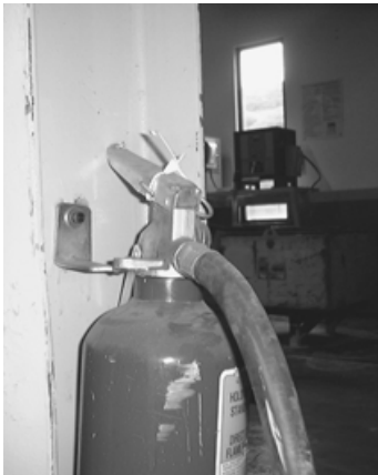
FIGURE 7.55 Extinguisher with damaged pin.
