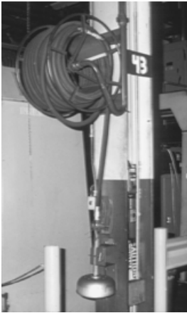
FIGURE 6.89 Carbon dioxide system hand line.
