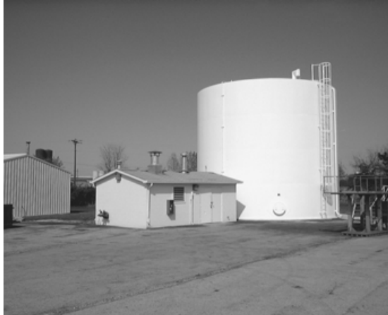
FIGURE 6.65 Suction tank and pump house.
