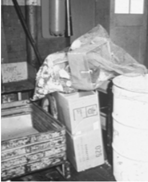
FIGURE 7.49 Obstructed access to extinguisher.
