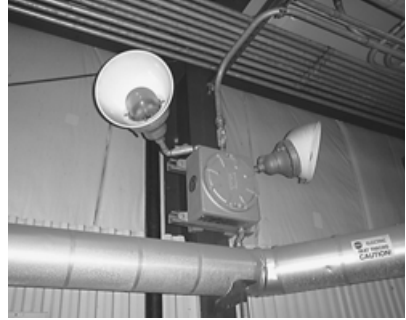
FIGURE 4.13 Emergency lights for a hazardous location.
