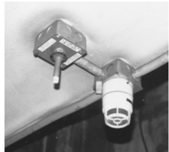
FIGURE 6.20 Smoke and heat detector.
