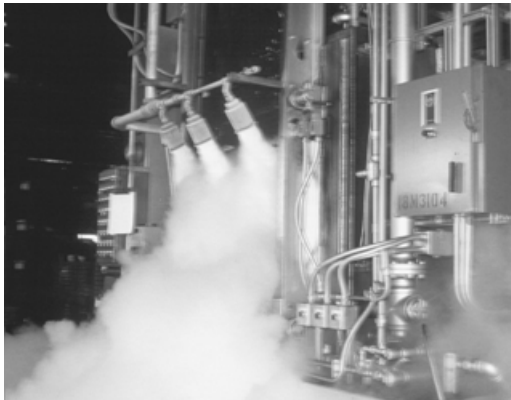
FIGURE 6.90 Carbon dioxide system discharge.
