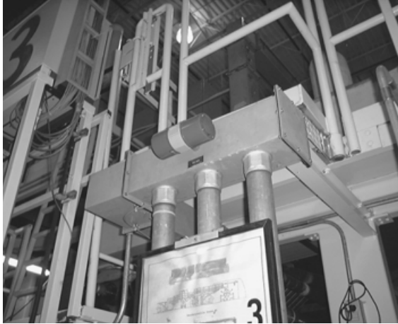
FIGURE 6.83 Carbon dioxide system pre-discharge alarm.
