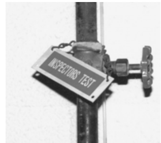
FIGURE 6.56 Inspector's test valve.
