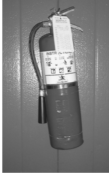
FIGURE 7.52 Extinguisher cylinder damaged.
