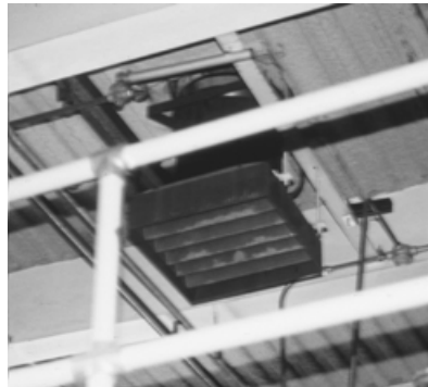
FIGURE 6.62 High expansion foam generator installed in roof.
