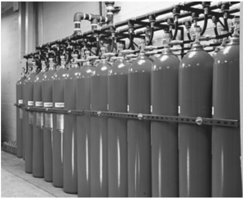
FIGURE 6.96 INERGEN® system. (Photo courtesy of Ansul Incorporated.)
