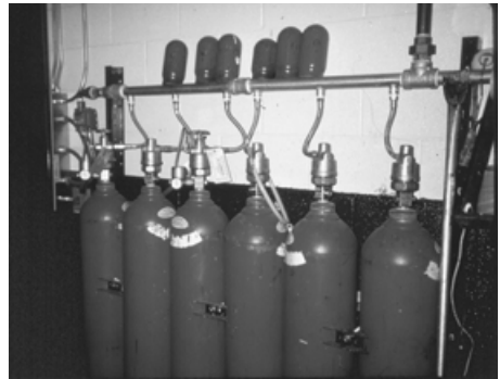
FIGURE 6.80 Carbon dioxide system high-pressure storage.
