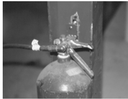
FIGURE 7.54 Extinguisher with missing pin.
