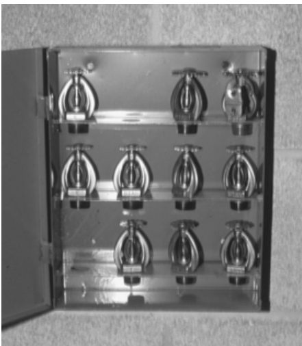
FIGURE 6.53 Extra sprinkler head cabinet.
