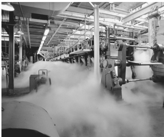
FIGURE 6.91 Carbon dioxide system discharge.
