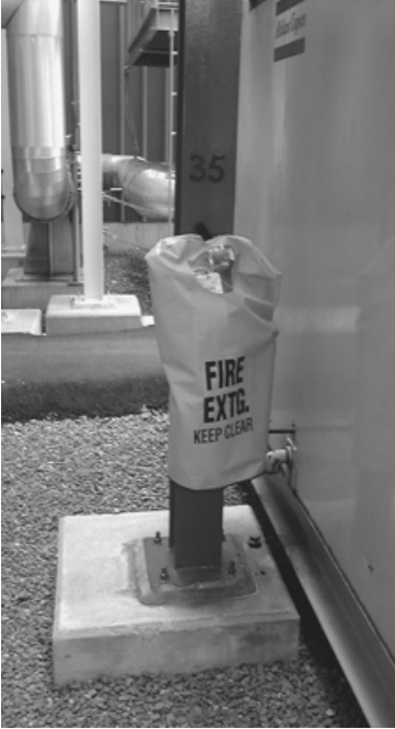
FIGURE 7.40 Extinguisher mounted outside.
