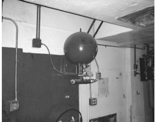
FIGURE 6.93 Halon system agent storage sphere.
