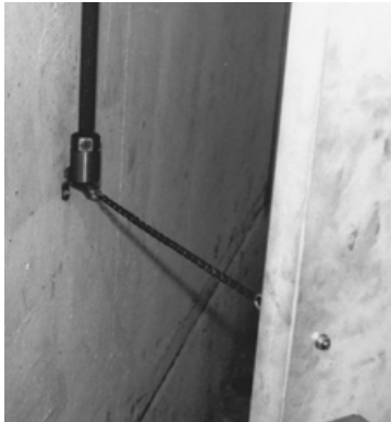
FIGURE 6.85 Carbon dioxide system door closer.
