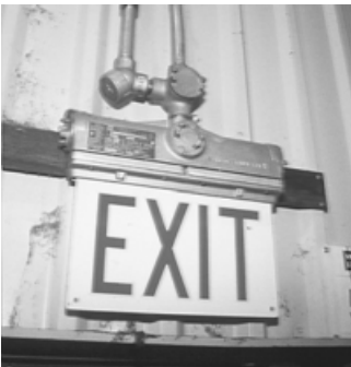
FIGURE 4.10 Exit sign for hazardous location.
