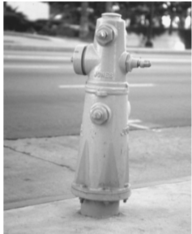
FIGURE 6.76 Wet barrel hydrant.
