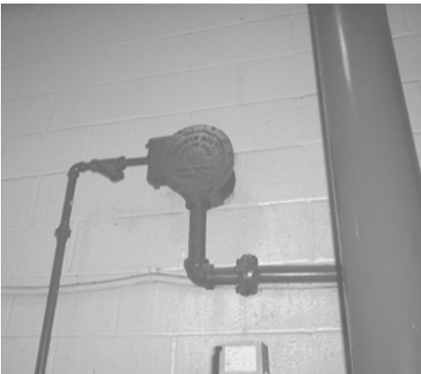
FIGURE 6.36 Water motor gong, inside building.
