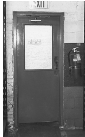
FIGURE 4.11 Door marked “not an exit.”
