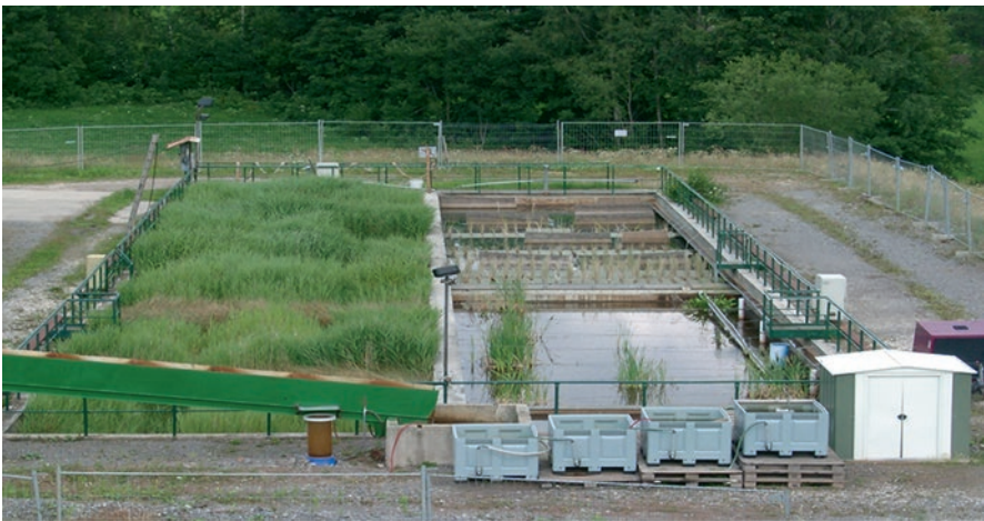
Fig. 9.17 Wisnut-designed mine water treatment system with rooted plants receiving water from the right side for treatment. On the right side, in the open water, Boojum recommended installing curtains for biofilm formation and floating cattail islands to address fine iron particles. In the foreground some cattail islands grew well, but others were plagued leaf lice. The light blue buckets were installed to provide a flow-through system for Chara . Growth data were used to derive design criteria for scale-up
