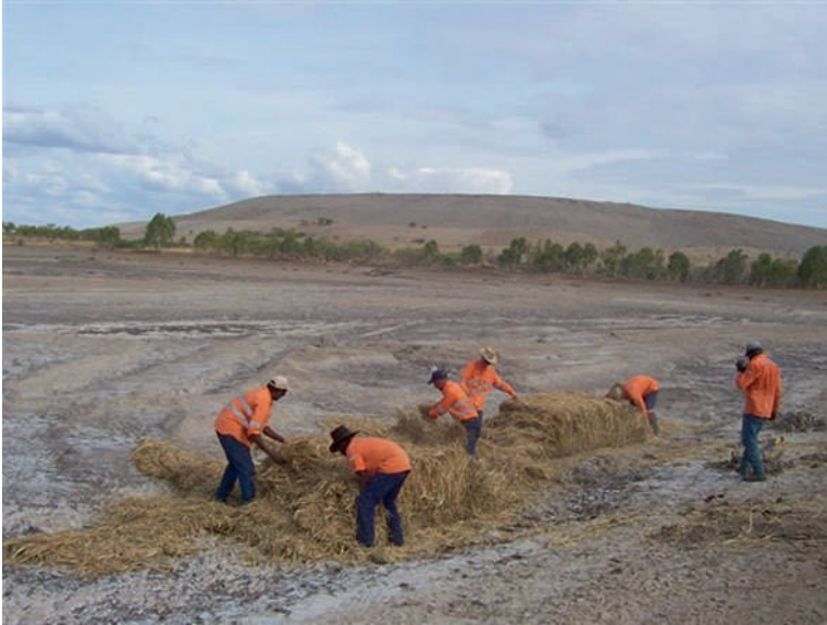
Fig. 6.1 Evaporation pond in northern Queensland, Australia, with straw bales being distributed prior to the monsoon season. (Photograph supplied by Century Mine)
